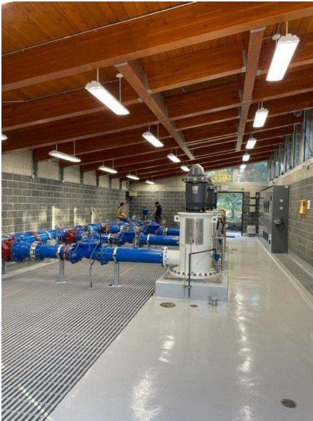
VICARRO PUMP STATION,
