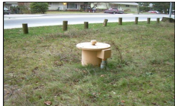
Groundwater Well Head
