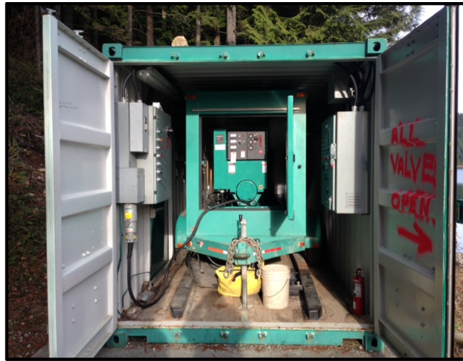
Photo 2 - Generator inside Sea Container
