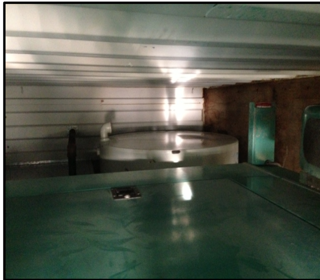
Photo 3 - Double-Lined Diesel Tank
